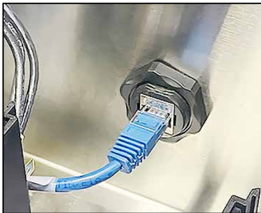
Fig. 4 - Ethernet port - Champion RJ45 from router (viewed from inside rear of control cabinet)
